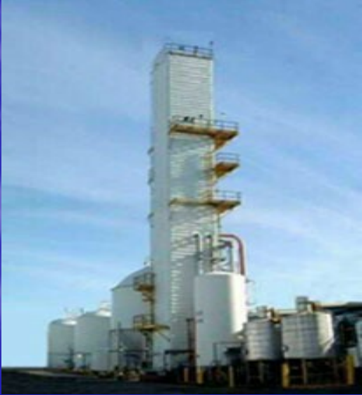
ZEROS Air Separation Unit
